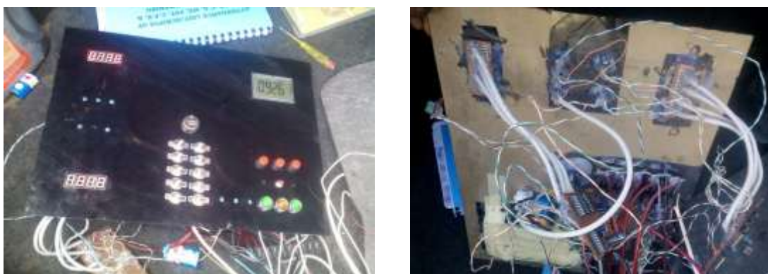
Figure 8: Panel controller for the CFB riser-regenerator systems awaiting installations
